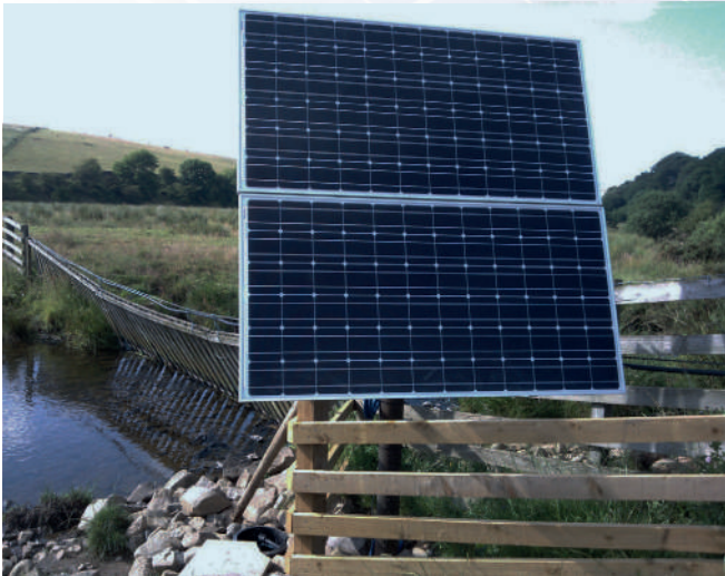
Figure 5: Solar panels used to power a pump.
