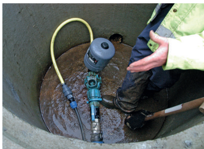
Figure 11. Ram pump within pumping chamber.
