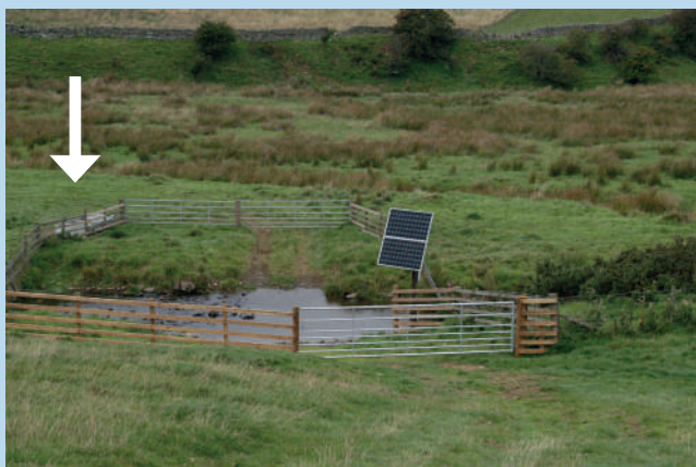
Figure 10: Solar System. The arrow shows secondary trough across watercourse. Primary trough installed in nearside field to right but out of shot.
