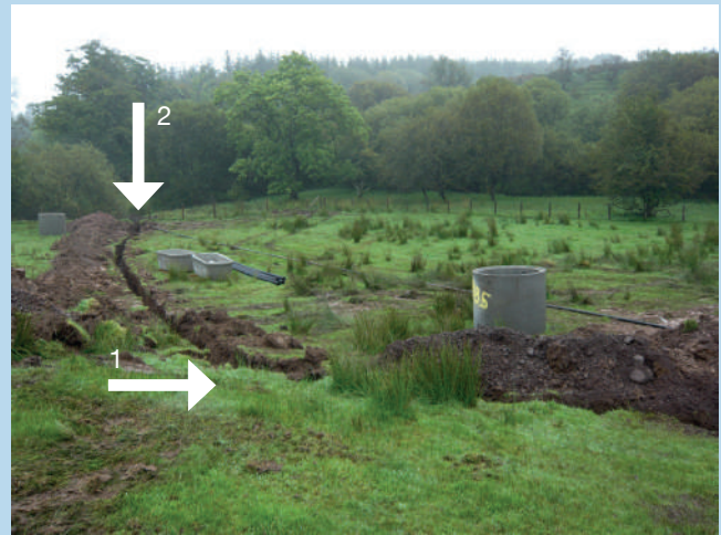
Figure 12: During installation. Note the site for the intermediate break chamber (1) and location of pump and discharge to watercourse (2). Abstraction point is 130m behind photographer.
